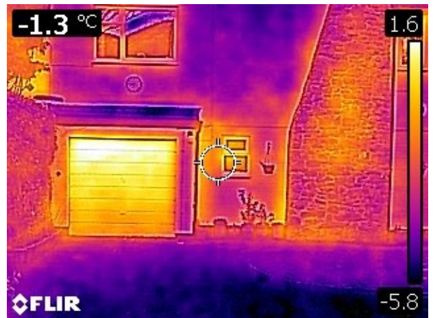
Thermal image of a local home. The yellow shows the warmer areas which may be sources of heat loss.
